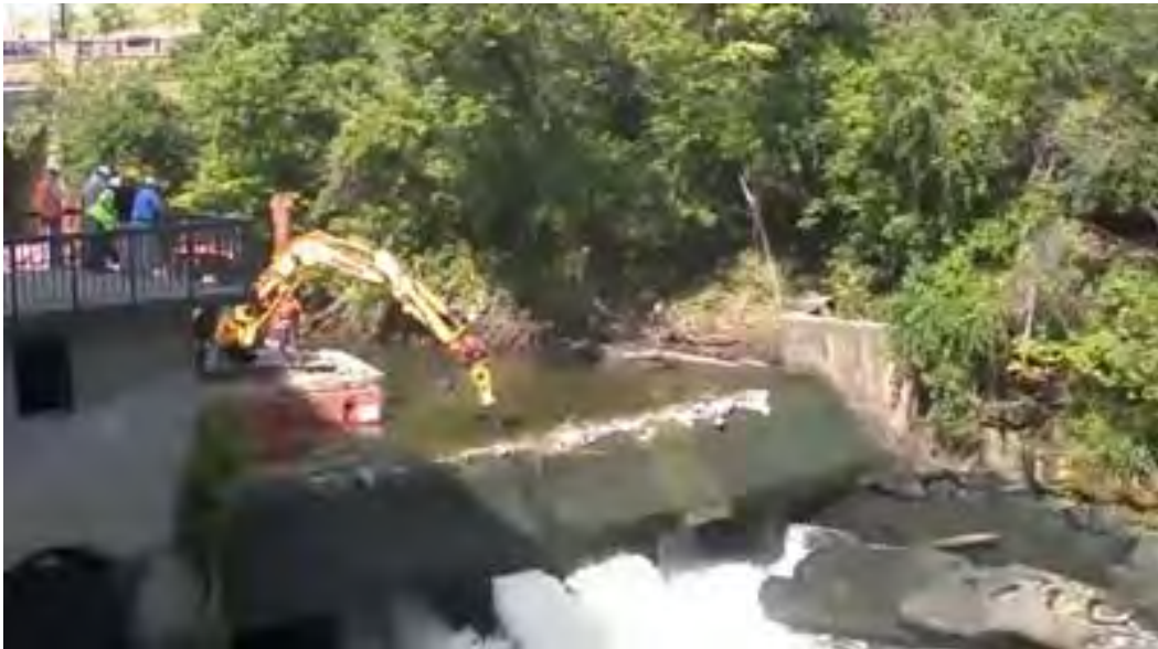
The dam is breached.
